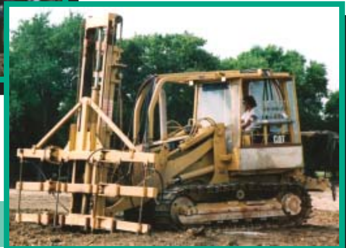
Injection unit shown on right is capable of injecting 30,000 square feet per day to a depth of 7 feet.
